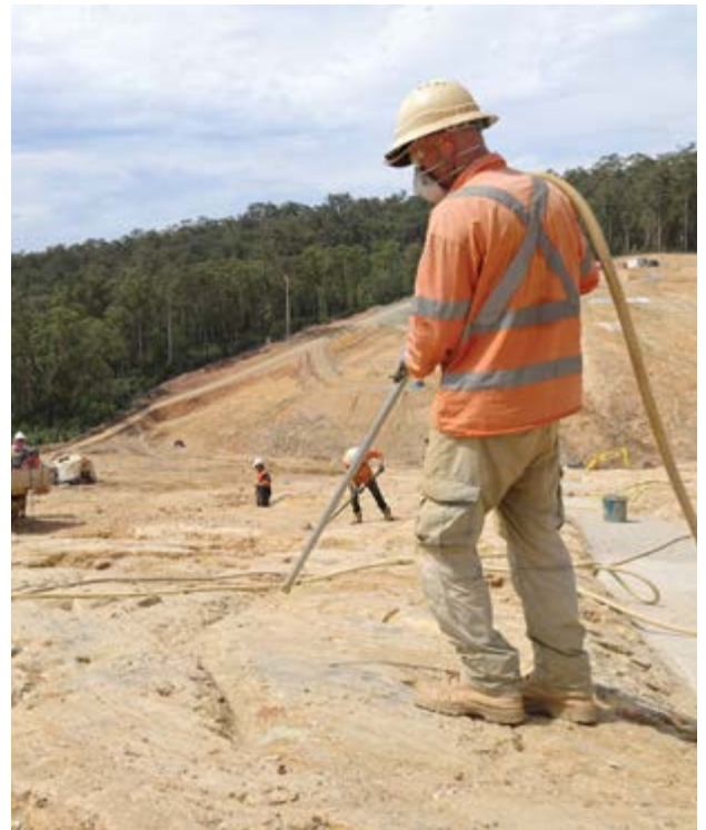
Image: Construction of the Southern Water Supply Storage/Dam is estimated to be 67% complete.
