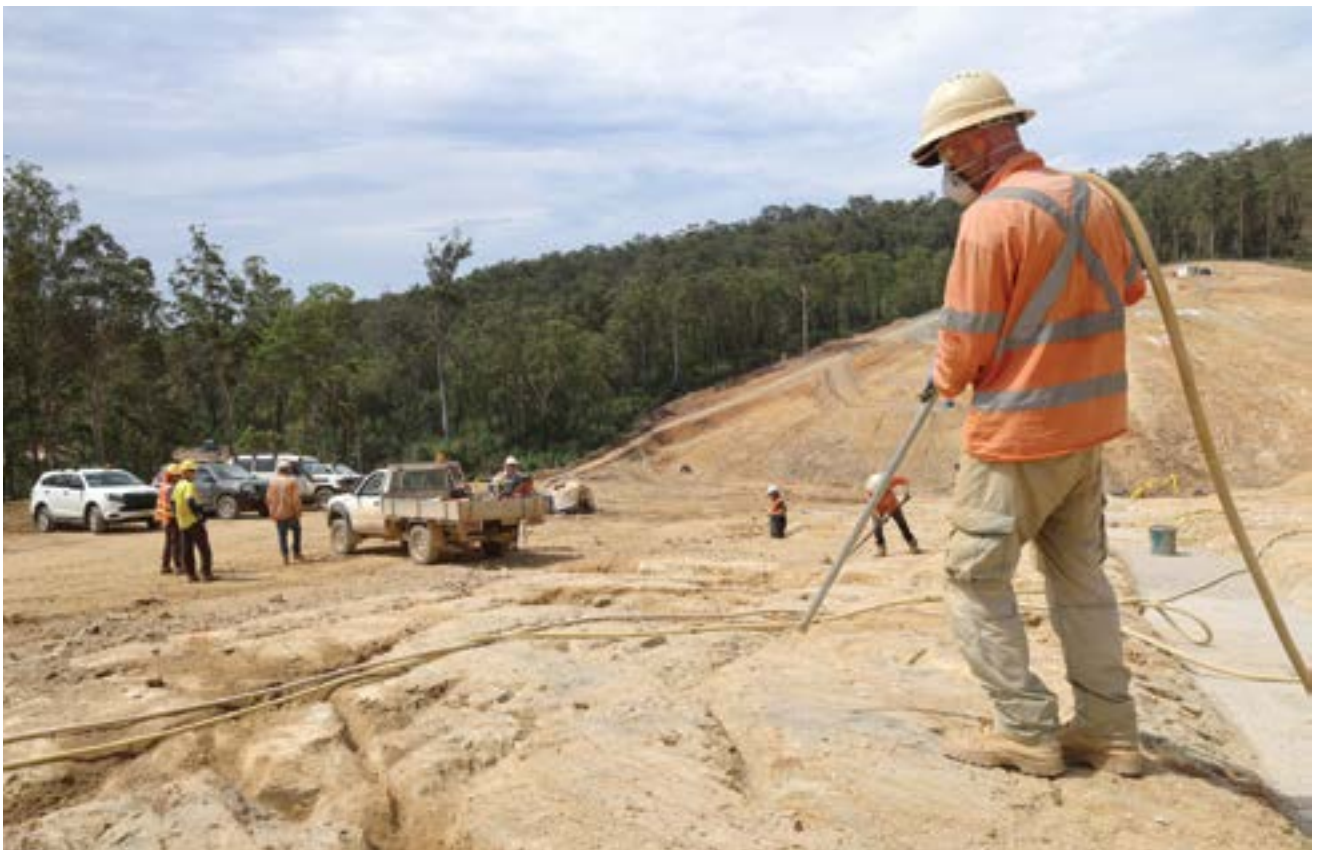
Image: Crews clean out a seam of the new dam wall foundation with high pressure air.
