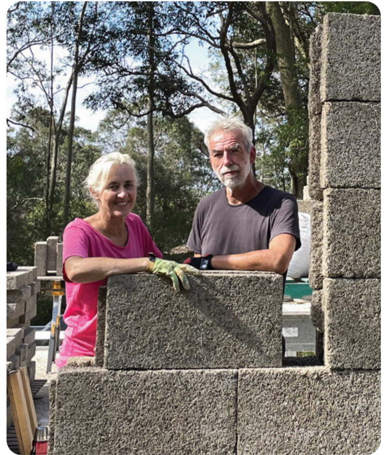
PROACTIVE: Kirsten and Dom Pitot are building their own sustainable home using blocks made of hemp.
